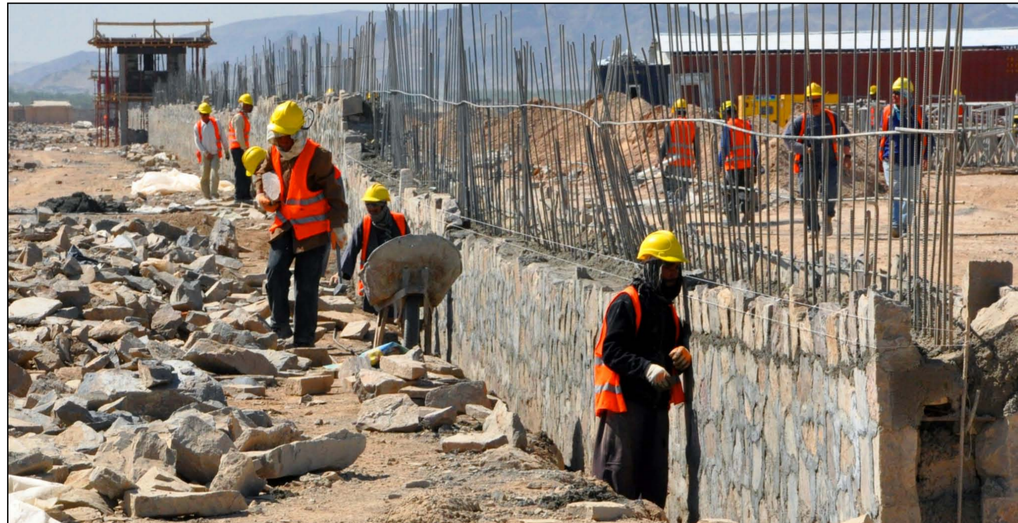
Progress continues on construction of the future home of the 3rd Brigade, 205th Corps Afghan National Army. As of April 19, the project was about 15 percent complete and will accommodate 6,000 ANA personnel. (USACE Photo by Jasmine Chopra-Delgadillo)
